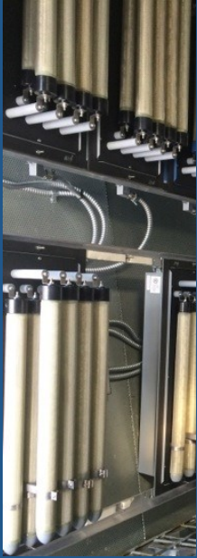
AtmosAir Model 500FCs rack-mounted systems in an AHU.
